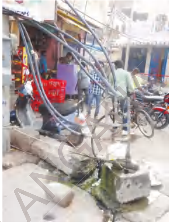
Fig. 14.6: Pipe lines for drinking water (Akasha Ganga)
